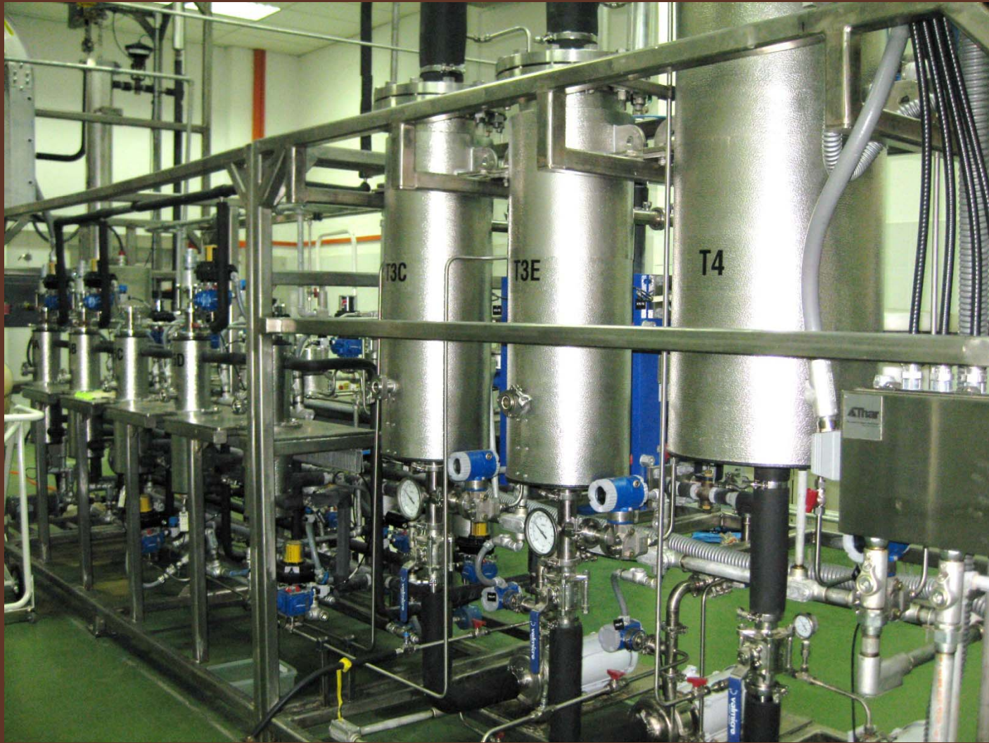
Separators and Flash Evaporators
